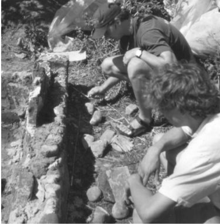
Figure 3. A small cobblestone wall under construction. Note the “backing stones” that form the back of the wall and the line of cobbles along the front. In between is the “trough” which will later be filled with rubble and mortar in advance of starting the next course.
