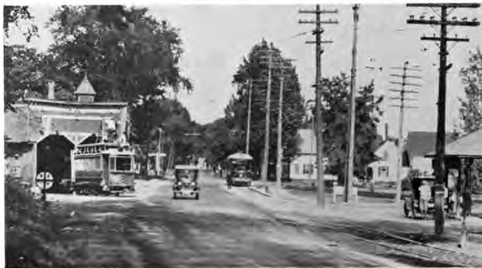
AFTER its passenger-carrying days were over, No. 16 was converted to a line car and as such is shown here with its crew working on the overhead at the Fairfield carbarn.
