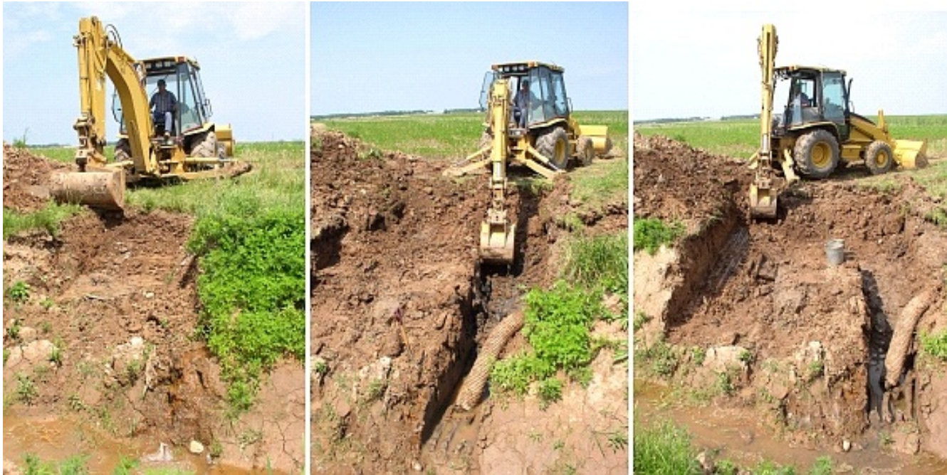
FIGURE 8: Three photographs showing the progress of mechanical excavation (left to right) to determine the extent of the in situ sluice (camera facing north).
