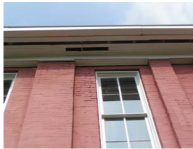
Front Soffit Deterioration
