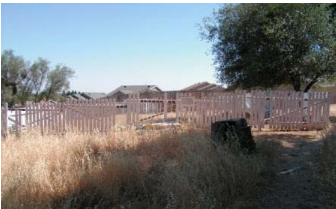
Skinner Ranch Cemetery Before the Most Recent Repairs to the Fencing.
